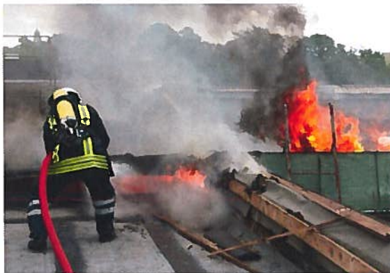
Fire caused by roofing operations
