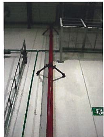
Sprinkler riser with sway bracing
