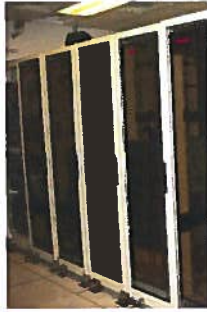
Computer server racks anchored to the floor
