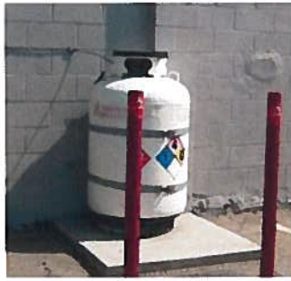
Flammable liquid tank strapped to wall
