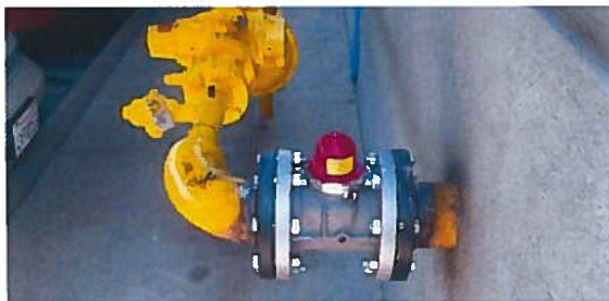
Seismic shutoff valve for natural gas line
