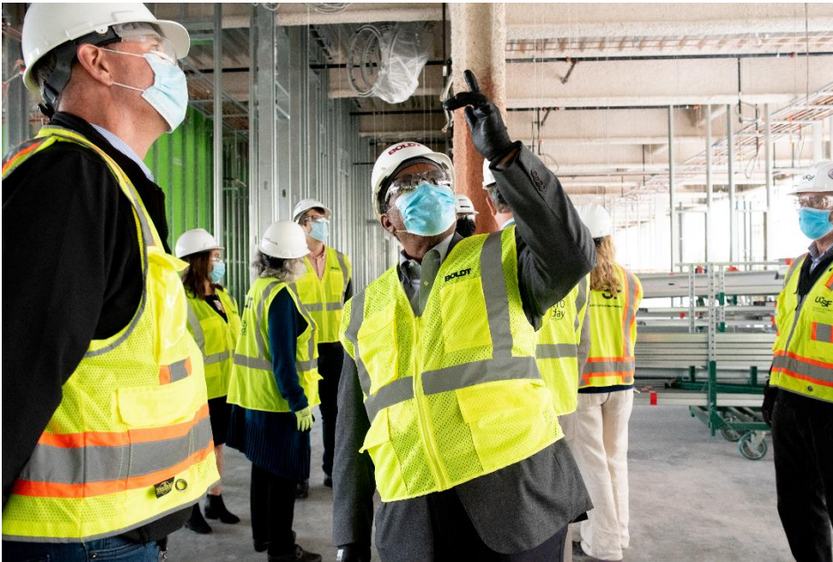
Photo: Construction walk at UCSF Research and Academic Building at Zuckerberg San Francisco General Hospital Credit: Barb Ries
